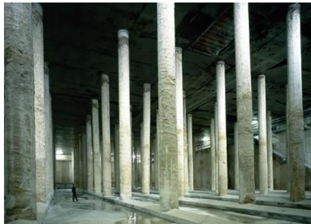
Fig. 08. Rainwater retention tanks
