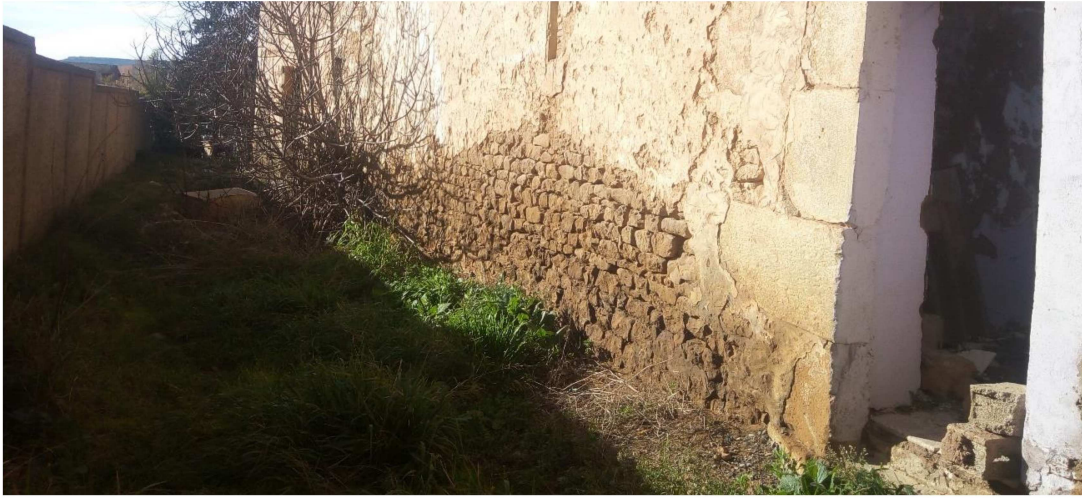
Figure 128: Remontées capillaires, façade extérieur est.
