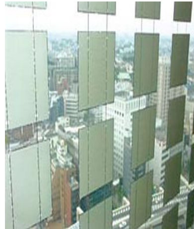
Figure 33: les panneaux photovoltaïques sur la façade du Yokohama Dia building (source: https://www.mitsubishi-logistics.co.jp )
